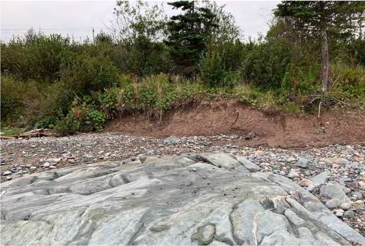
Figure 29. Clay bed with pipe on surface slump. Facing north at waypoint 171.
