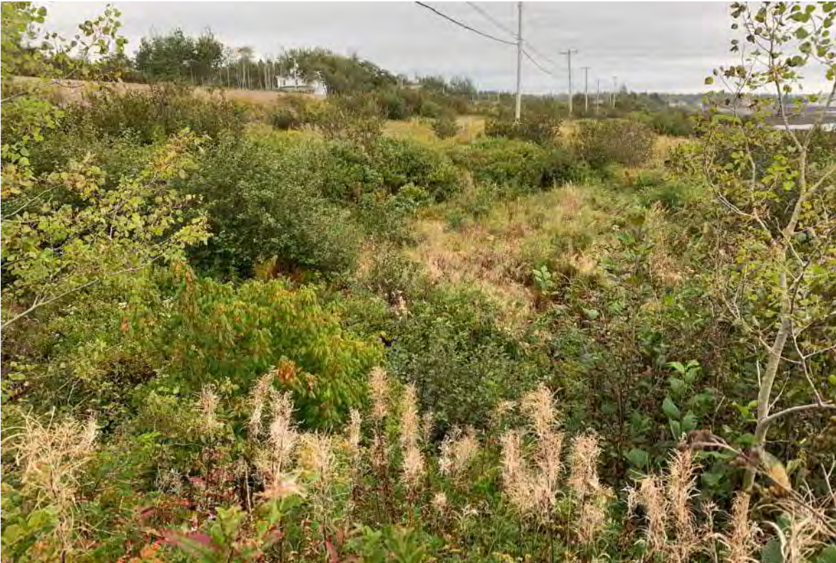
Figure 43. Facing east from waypoint 175, steep, 5 m bank to drainage channel for culvert under roadway.
