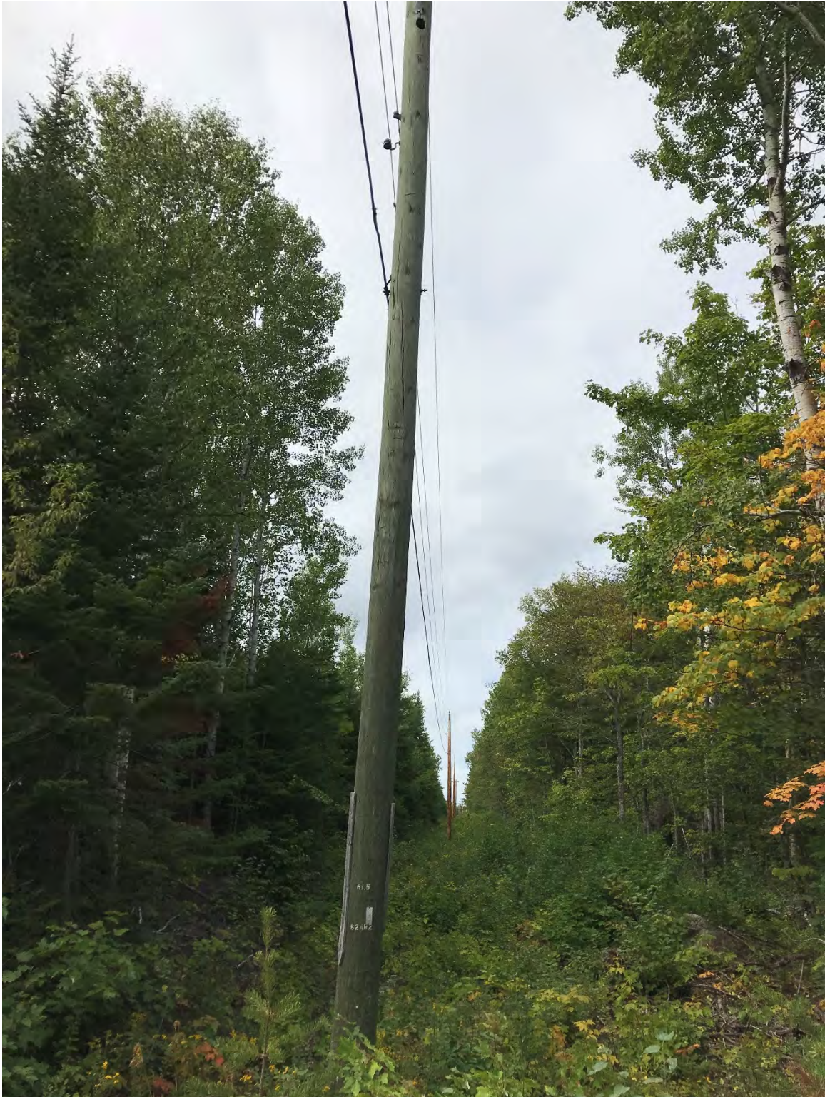
Figure 22. Photograph looking northwest showing the 12 kV power line easement between an NB Power transformer and NB Route 430 at Brunswick Mills, New Brunswick.
