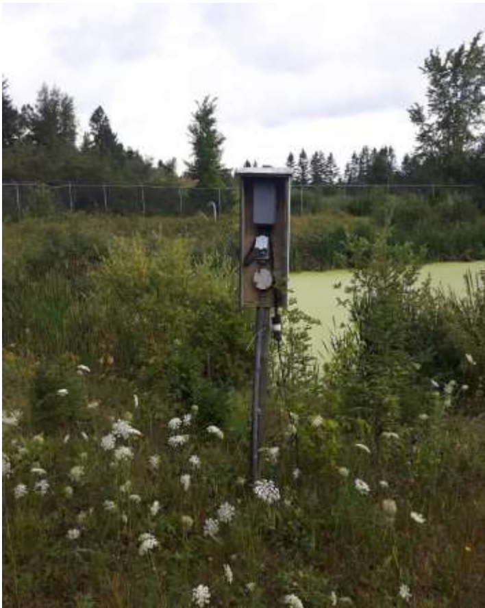
Photo No. 3: Electrical Entrance and Chemical Disinfection (in background)
