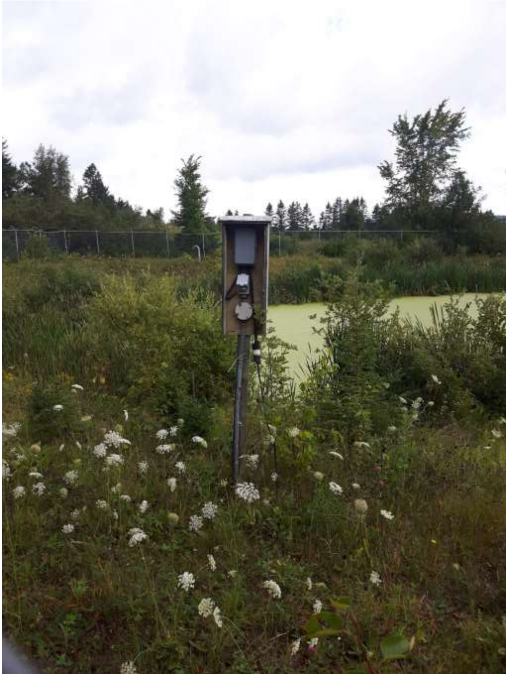
Photo No. 7: Lagoon Electrical Entrance
