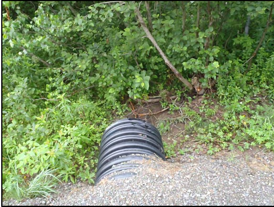
Photo 11 – Dry upstream side of culvert in the eastern part of the Site.
