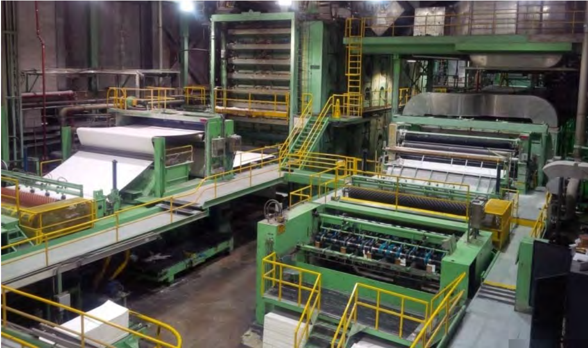
Figure 5. Photograph showing the existing #1 and #2 pulp dryers at the Reversing Falls Mill in Saint John, New Brunswick.
