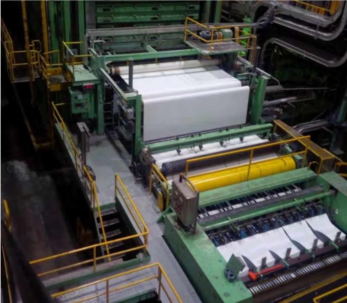
Figure 6. Photograph showing the existing #3 pulp dryer at the Reversing Falls Mill in Saint John, New Brunswick.
