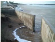
Erosion Control Structure Failure, Bathurst, NB
