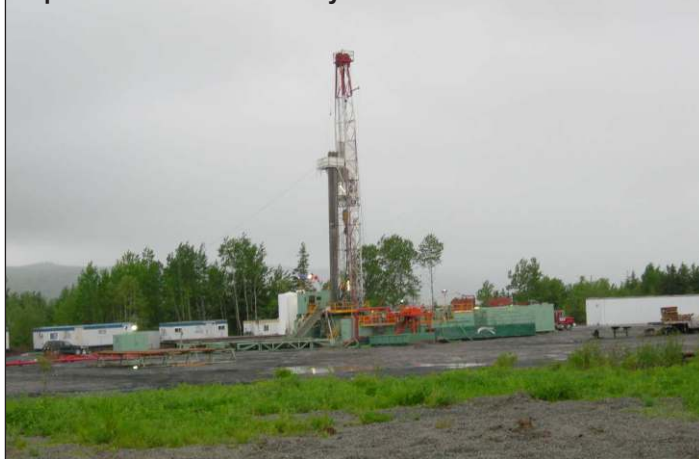
Drilling of the I-88 directional well (Well 749) of Contact Exploration Inc. in the Stoney Creek Field.
