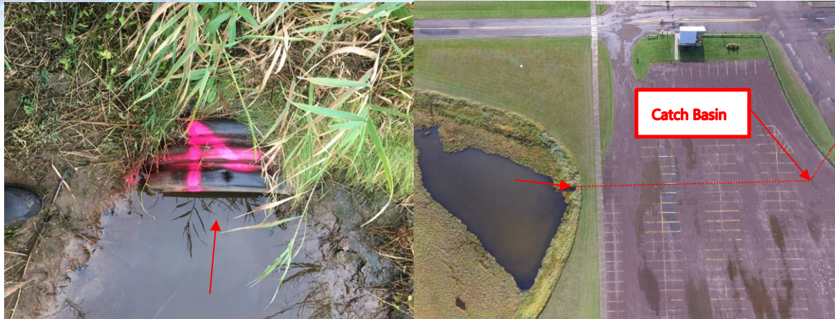
Figure 2-6: Storm Outlet No. 4 (450mm Diameter High-density polyethylene (HDPE))
