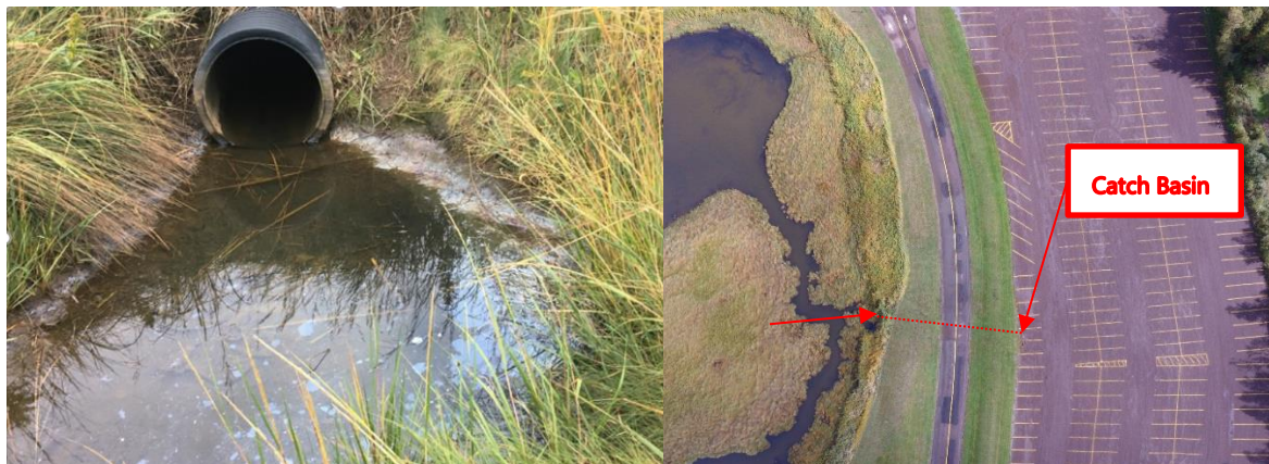
Figure 2-7: Storm Outlet No. 5 (600mm Diameter HDPE)
