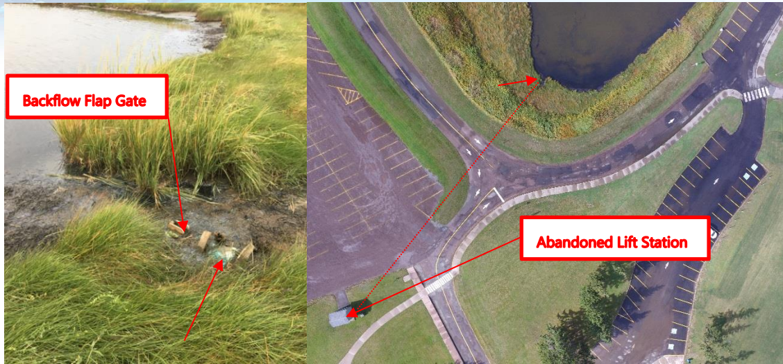
Figure 2-8: Sanitary Overflow No. 6 (250mm Diameter PVC)
